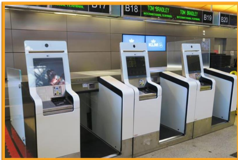
Terminal B Automated Bag-Drop System
