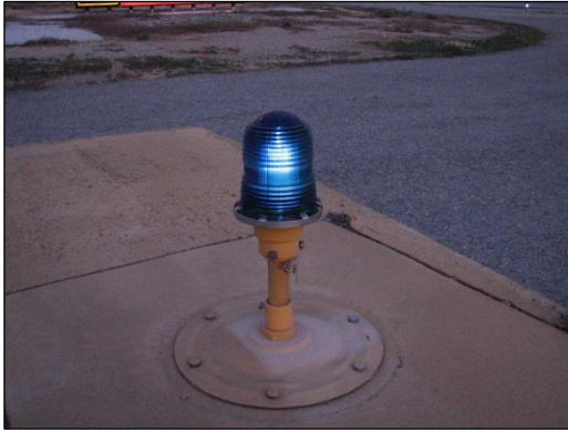
Taxiway Edge Light (elevated)
