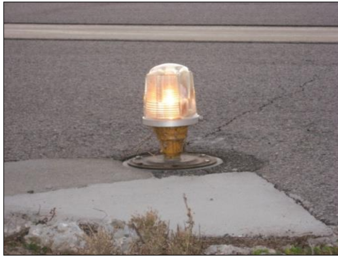
Elevated Runway Edge Light Fixture
